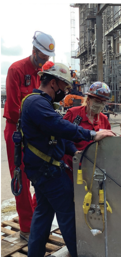
A contractor employee shows Parish President Matt Jewell and GM Tammy Little some of the equipment he is working on during the Rock Dat Turnaround.
